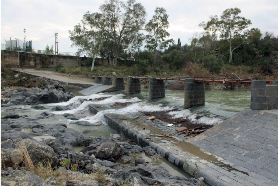
Figure 3. Santa Domenica water intake (Picture by anonymous)
