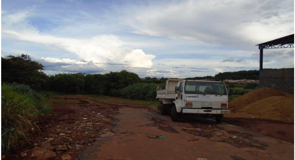
Figure 4: View of a dolina that opened in January and the intervention to cover it with earth in Vazante ( Personal Archive, 2022).
