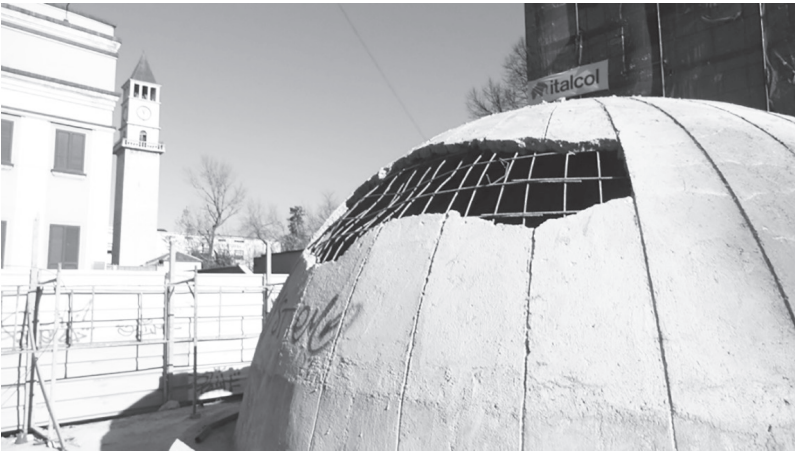
Fig.8 Dome damaged by protests
